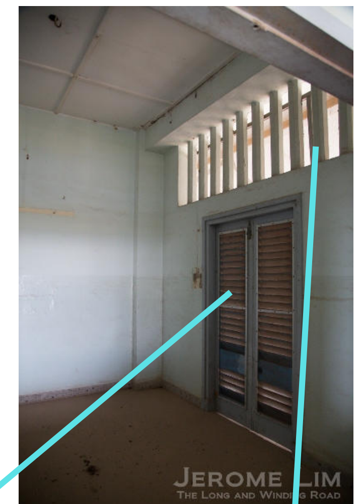
Concrete vents in the rooms for natural ventilations
